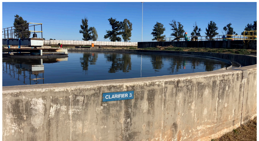
Matlosana Stilfontein Waste Water Treatment Plant
