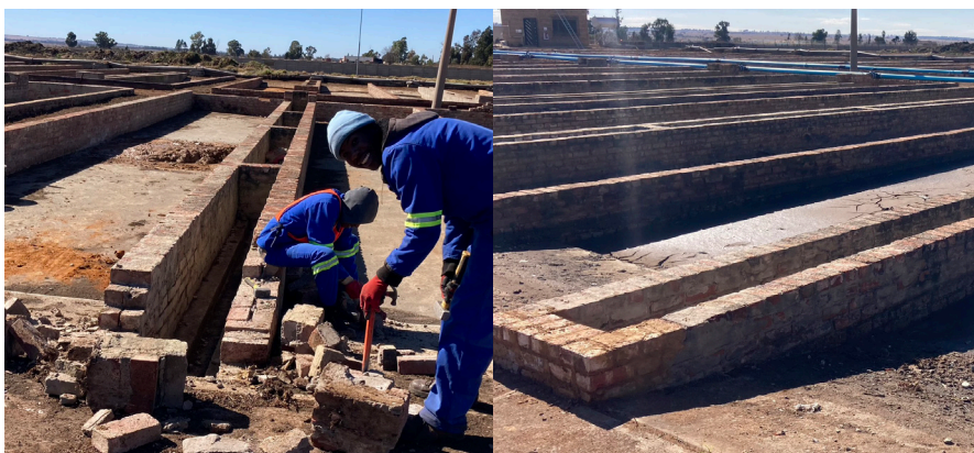
Merafong Oberholzer Waste Water Treatment
