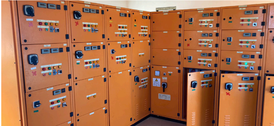
Matlosana Stilfontein Waste Water Treatment Plant
