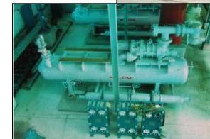
Surface Ice plant
