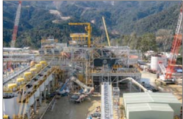
Hidden Valley – Sag Mill & Grinding Area
